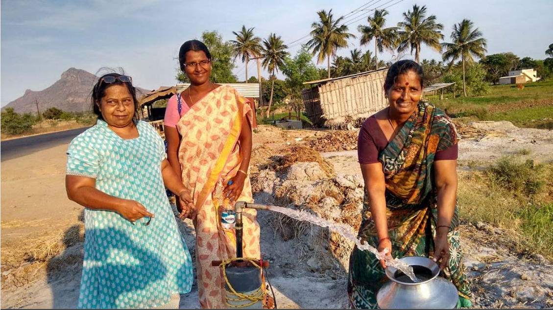
Digging of borewells with rigs and fixing electrical motors to draw water in 7 villages, Andhra Pradesh, India, project no. 0966.
